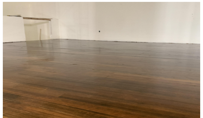
Level 1 Stage Floor Staining
